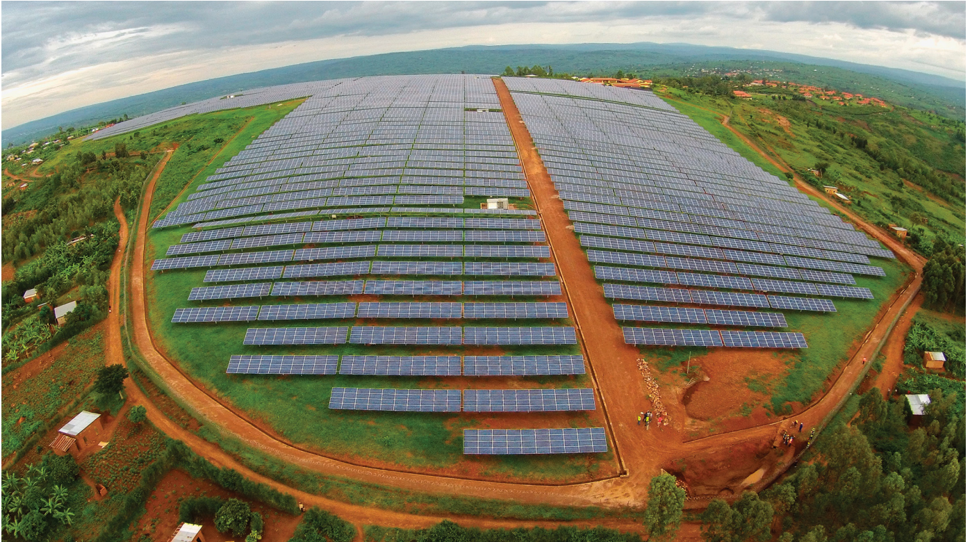
A $23 million project, the solar field at the Agahozo Shalom Youth Village outside of Kigali, Rwanda, was the first utility-scale, grid-connected, commercial solar field in East Africa. Photo credit: Flickr/Sameer Halai/USAID/Power Africa.
